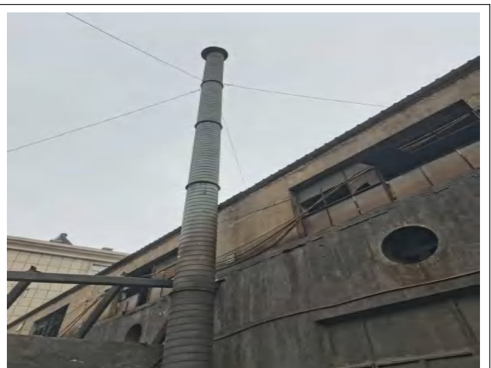
15M 废气排放塔
